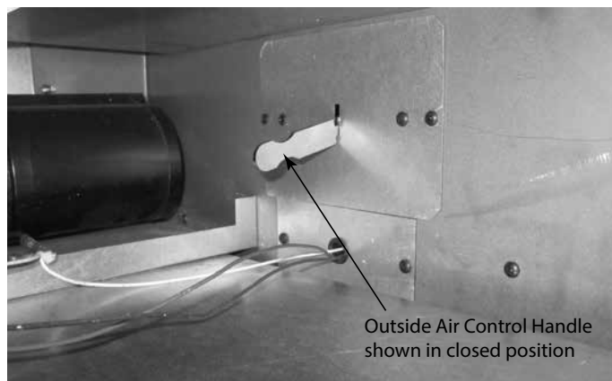
Figure 3.6 Outside Air Control Handle
